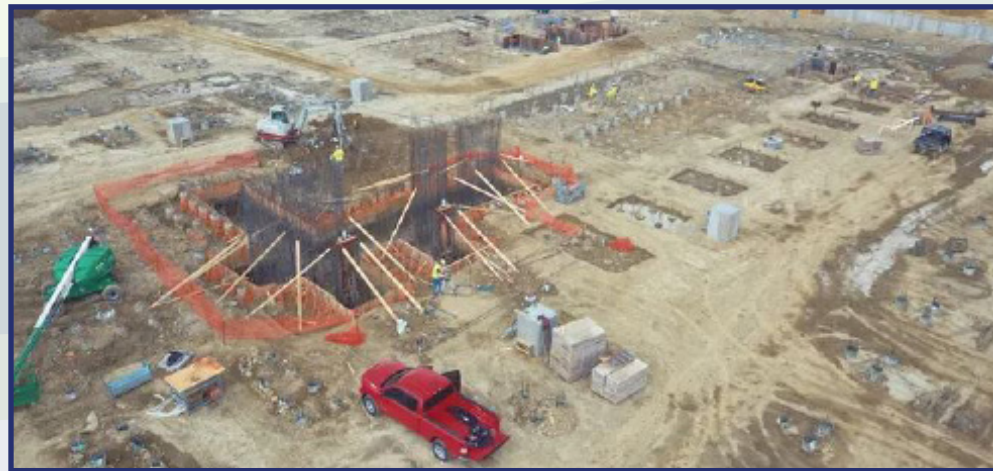
Construction at the Pratt Paper site in Henderson SOURCE: Henderson Economic Development
