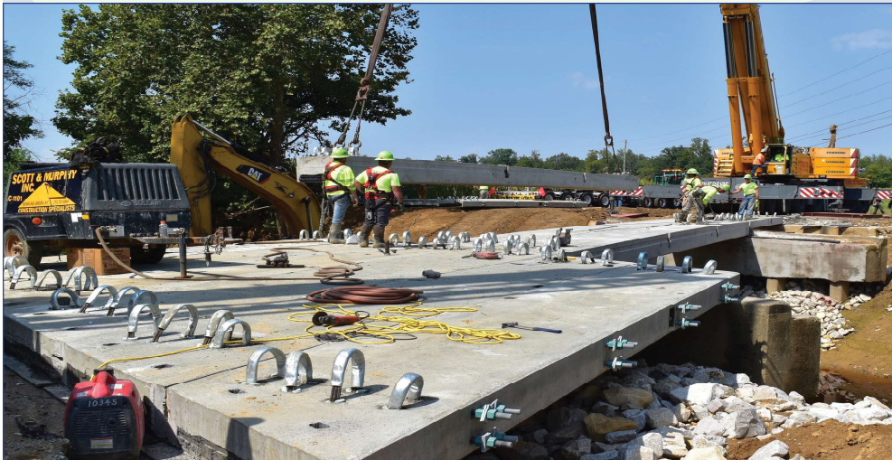
New beams are being installed for the Panther Creek Bridge Replacement Project on Old Hartford Road. (Photo/Daviess County Fiscal Court Facebook)
