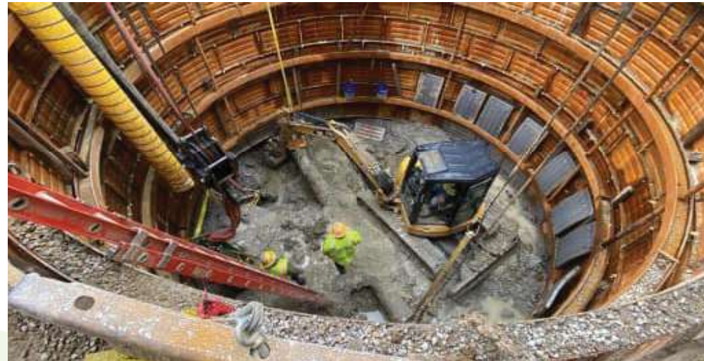
Construction takes place on the Ohio County Water District Intake Project. (Photo/GRADD)
