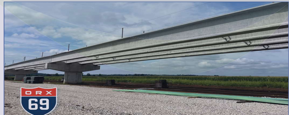
Beams installed at the Bridge Approach for the I-69 Ohio River Crossing. Each beam is 188 feet long and weighs over 100 tons. (Photo/I-69 Ohio River Crossing Facebook)
